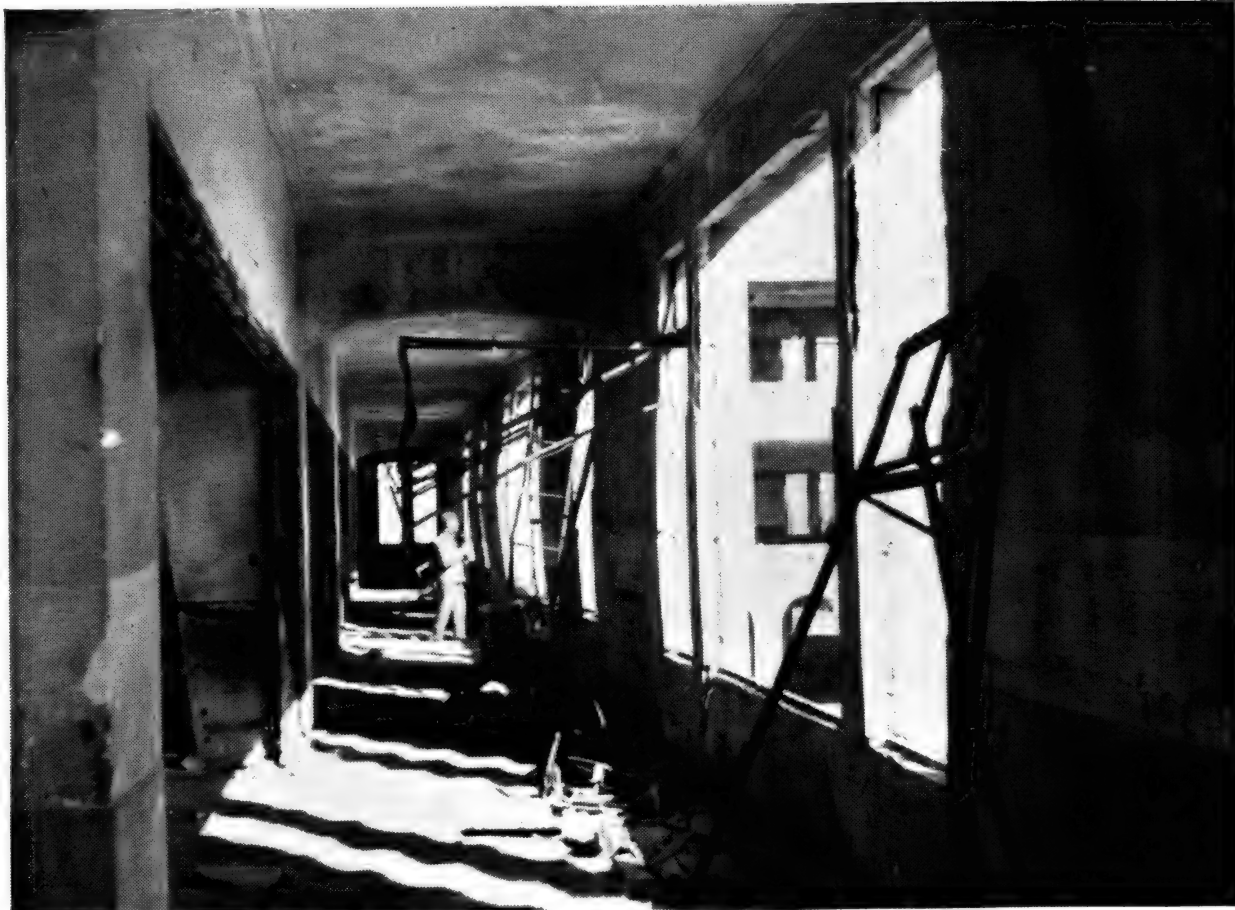
Photo No. 9. HIROSHIMA. Reinforced concrete school 500 yds. from the centre of damage, which is to the right. The frame of this building was of special design (portal) and resisted the lateral forces. The outside walls were of continuous reinforced concrete, and although they were deflected, as seen, they did not fail. See paragraph 27.
